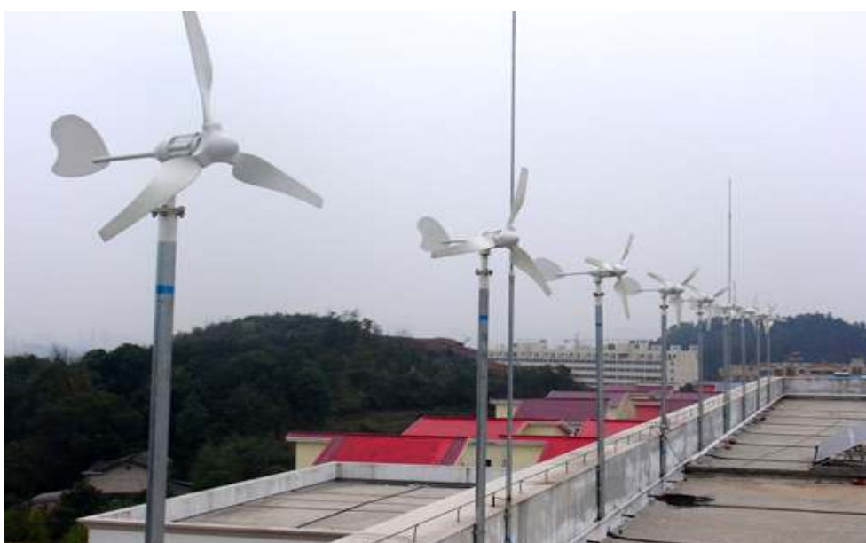
Actual Field Picture, Residential Lighting Power Supply System Installed on the Top of the Building, Royal View Residency.
