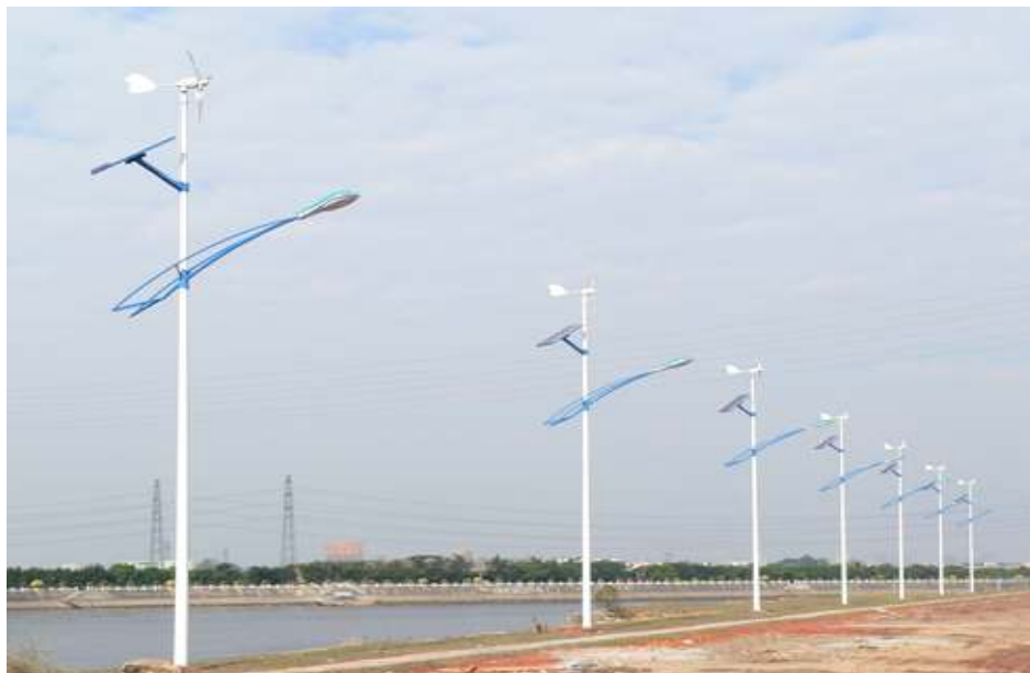
Roadside Wind/Solar Hybrid Lighting Power Supply System, International Bio-island
